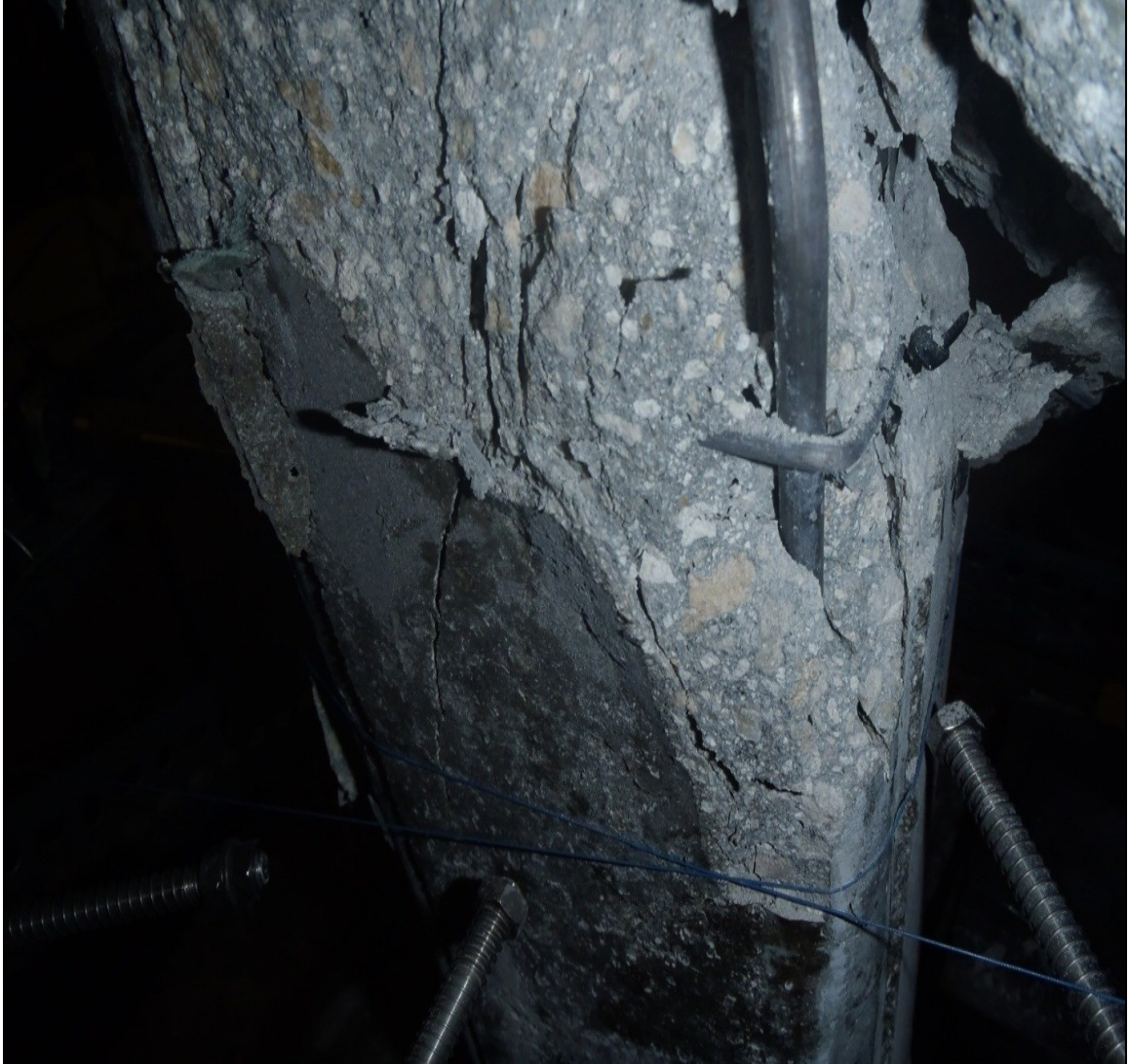
Fig. B-15: Failed control column
