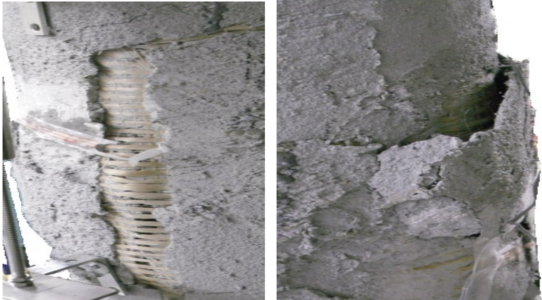
Fig. 4-4: Typical column element after testing
